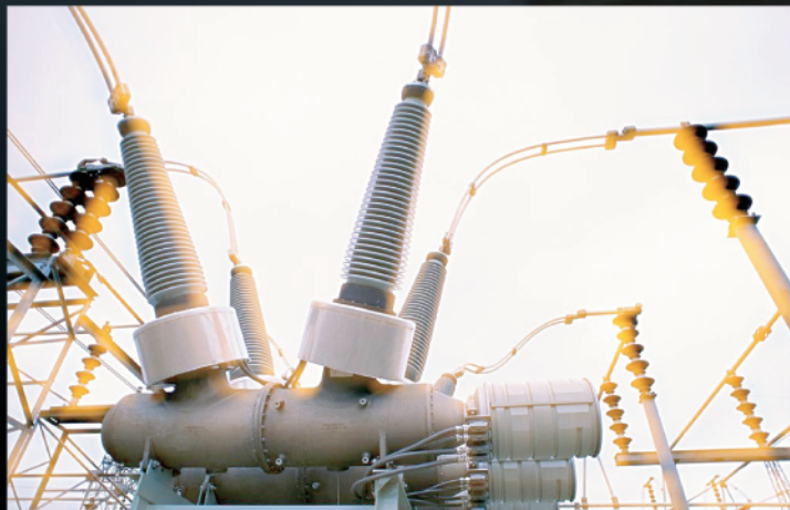
Transformer insulation material
